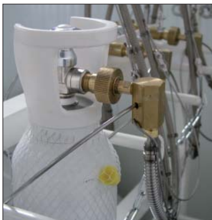
High pressure hose connected to the cylinder
